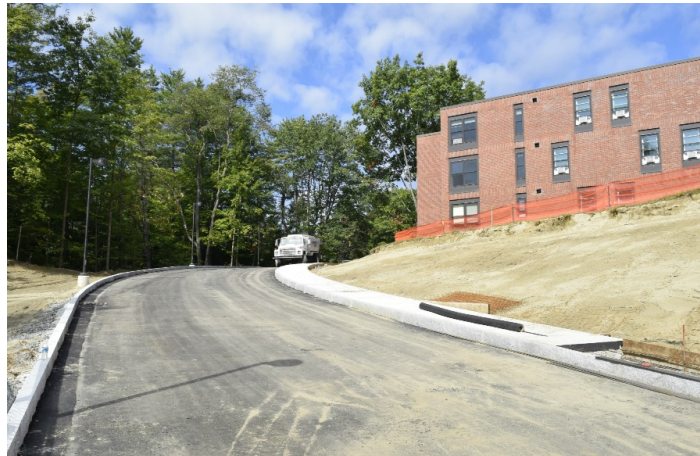
When the access road opens in early October, it will be called Thayer Drive.
