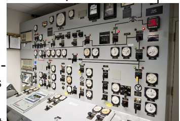
The control room panel
