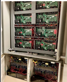
This shows some Intelligent System Controller circuitry that enables door access when you present your ID badge to a card reader
