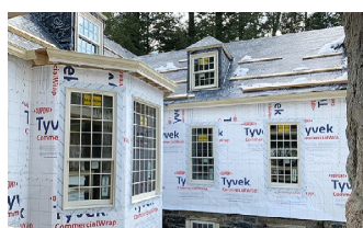
New bay windows have been installed between the main lounge and new dining room.
